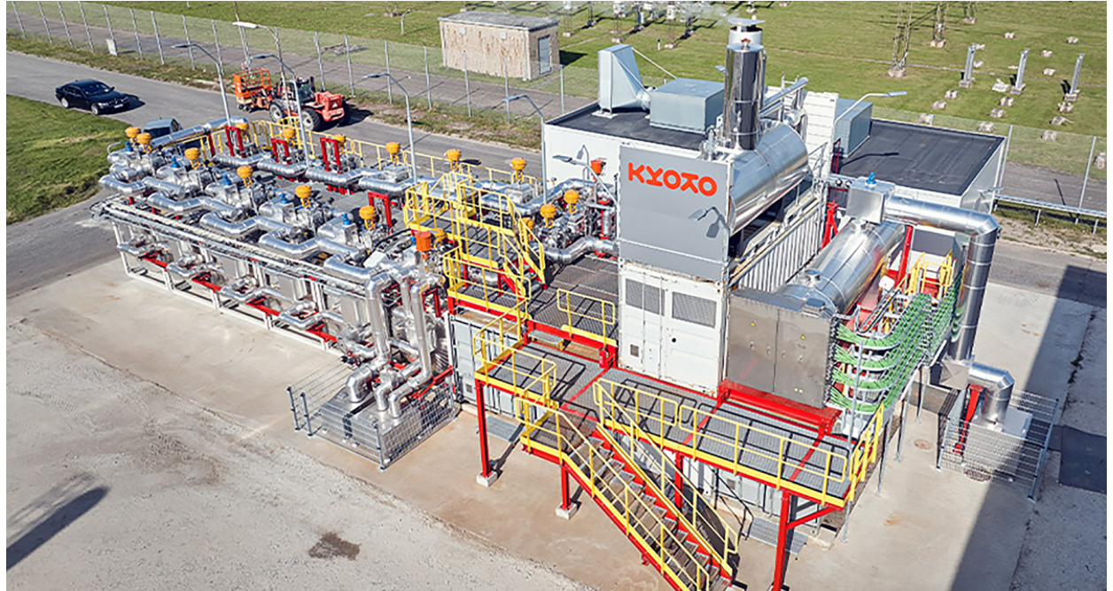
Fig. 3: Heatcube at Norbis Park has replaced coal for district heating in Aalborg, Denmark. It is charged with 5MW and has a storage capacity of 18 MWh. This Heatcube reduces emissions up to 2000 tonnes of CO 2 per year.
